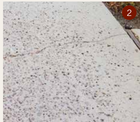
Scaling from freeze-thaw, chemical attack, poor quality concrete mix or improper finishing.
