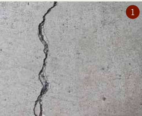
Cracking may indicate an unsound concrete substrate.
